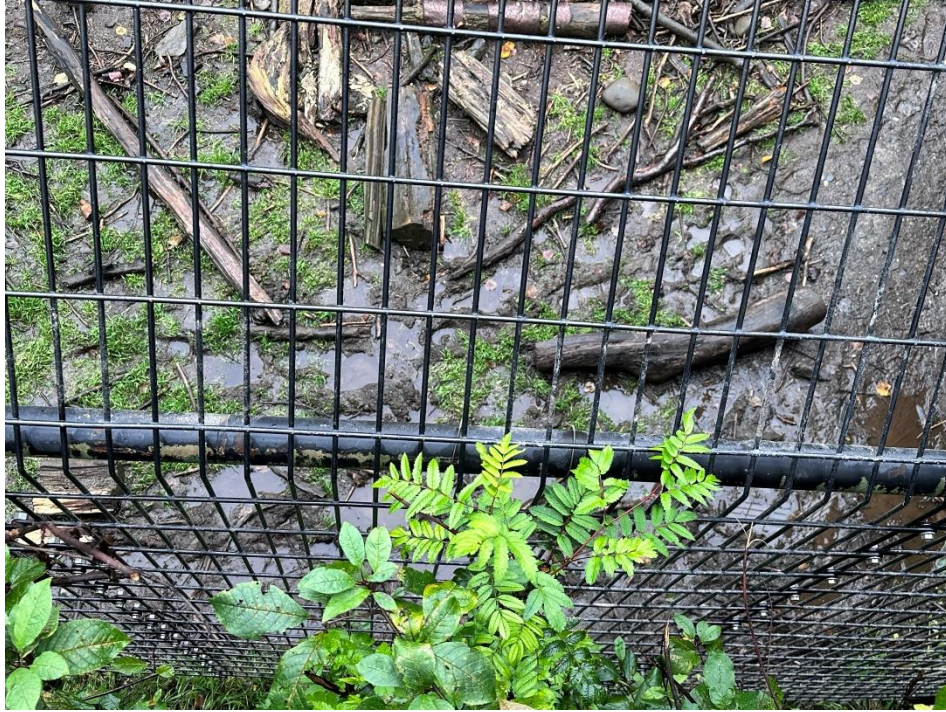
Figure 6. Lower fencing of black bear exhibit just above S. Fork Little Campbell Creek
